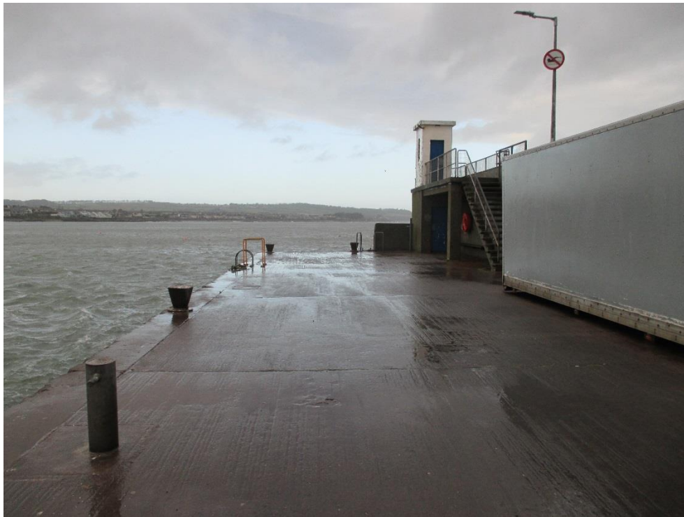
Fig B1 – View of the West end of the Piled Section of Pier
