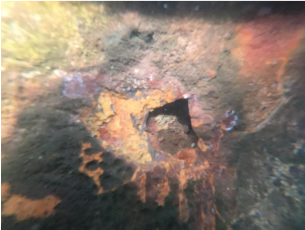
Fig B35 - Hole beneath Repair Plate at top of Outpan No. 173 – Very thin material surrounding repair
