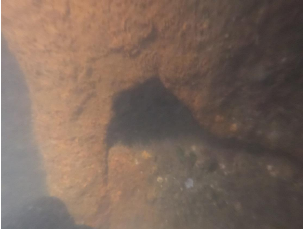
Fig B29 - Typical Hole in Pile at MLWS along South Face -
