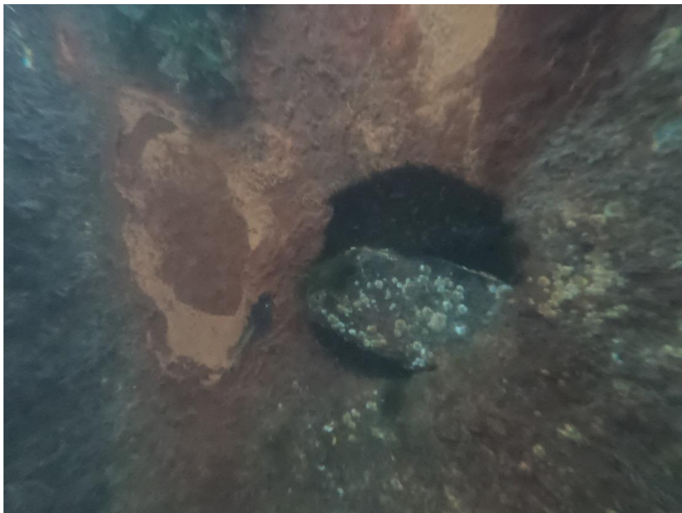
Fig B24 - Hole at MLWS, Outpan No. 119 – ALWC evident at same level.
