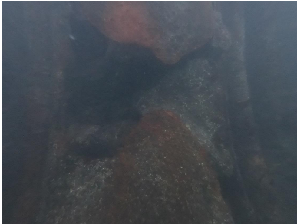
Fig B25 - Hole at MLWS, Outpan No. 117 – Typical at same level
