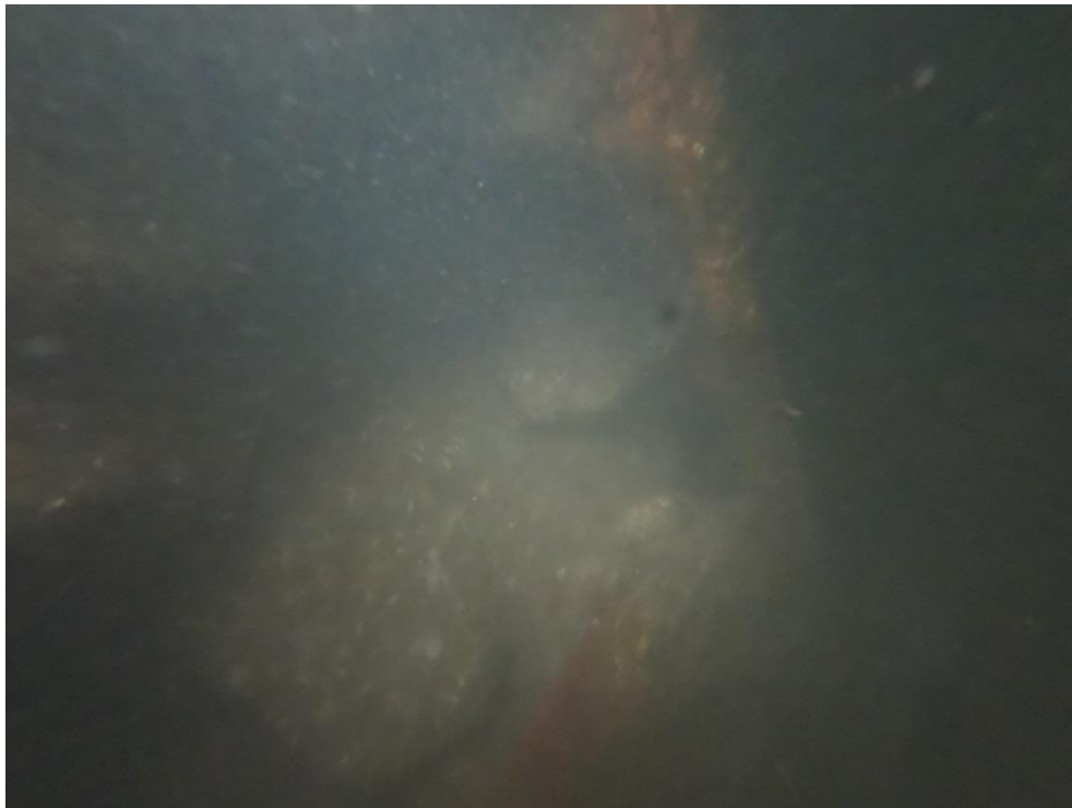
Fig B31 - Complete loss of Pan Face at Outpan No. 219 (Typical Elsewhere)
