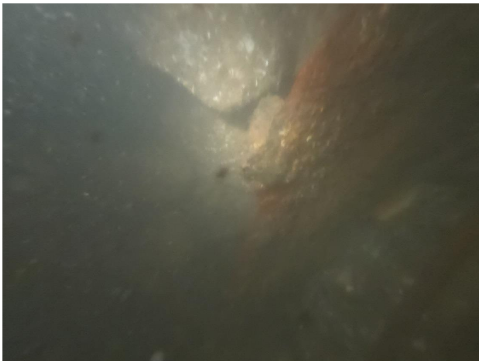
Fig B32 - Loose flap of Steel following loss of pan face – Typical
