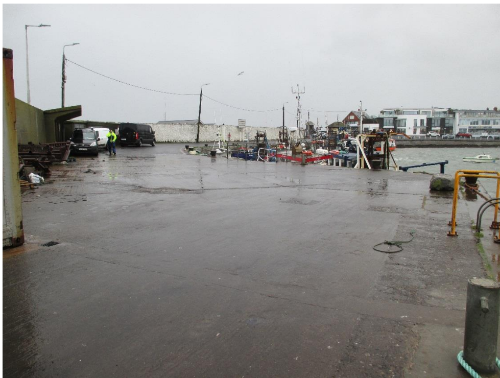
Fig B2 – View of the East end of the Piled Section at the interface with the Original masonry pier
