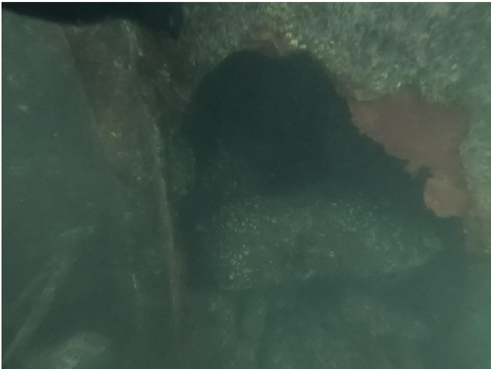
Fig B18 - Hole at bottom of Pile above MLWS – Outpan No. 13, Northeast Wing
