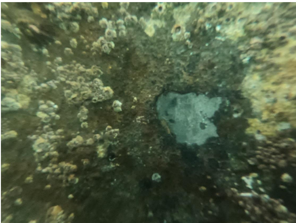
Fig B16 - Typical Steel Surface condition at lower Intertidal Zone (Corrosion removed for UT measurement)
