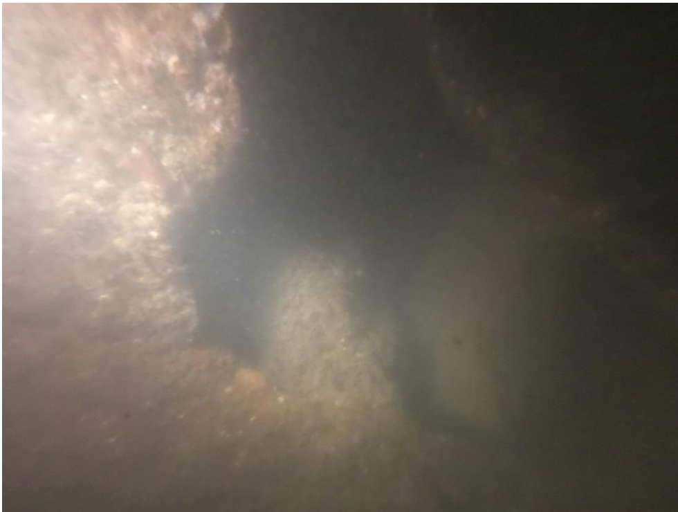
Fig B30 - Hole at Bed level – Outpan N0. 217 – Note Void behind
