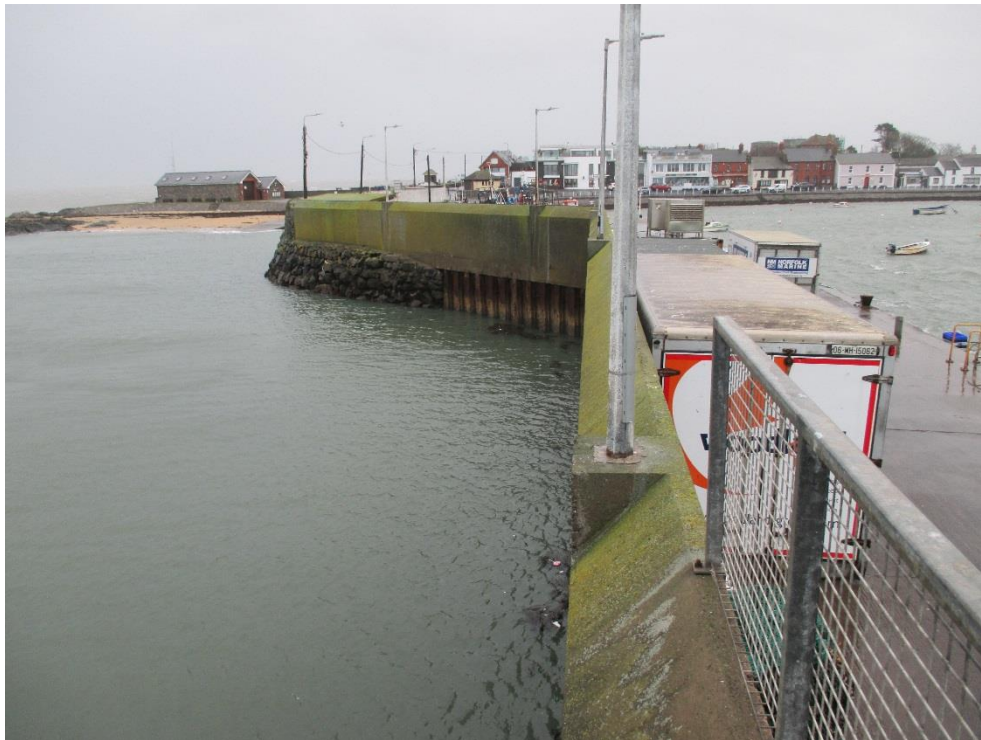
Fig B3 – View of the Northeast Wing of the Piled section (Start of Pile numbering)
