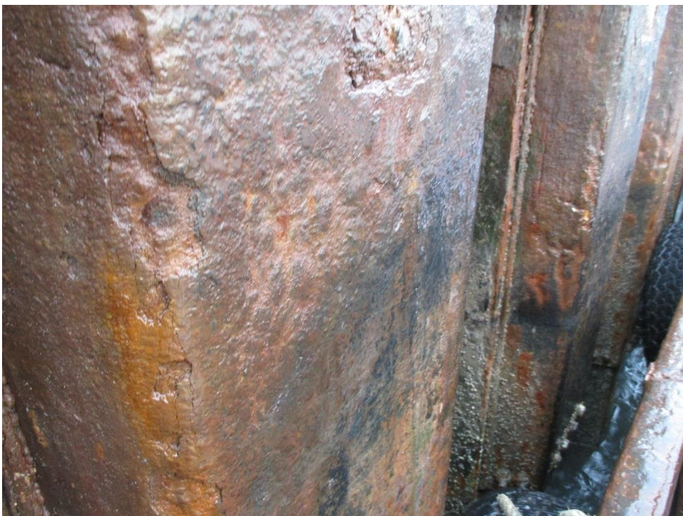
Fig B12 - Typical corrosion delamination and pitting
