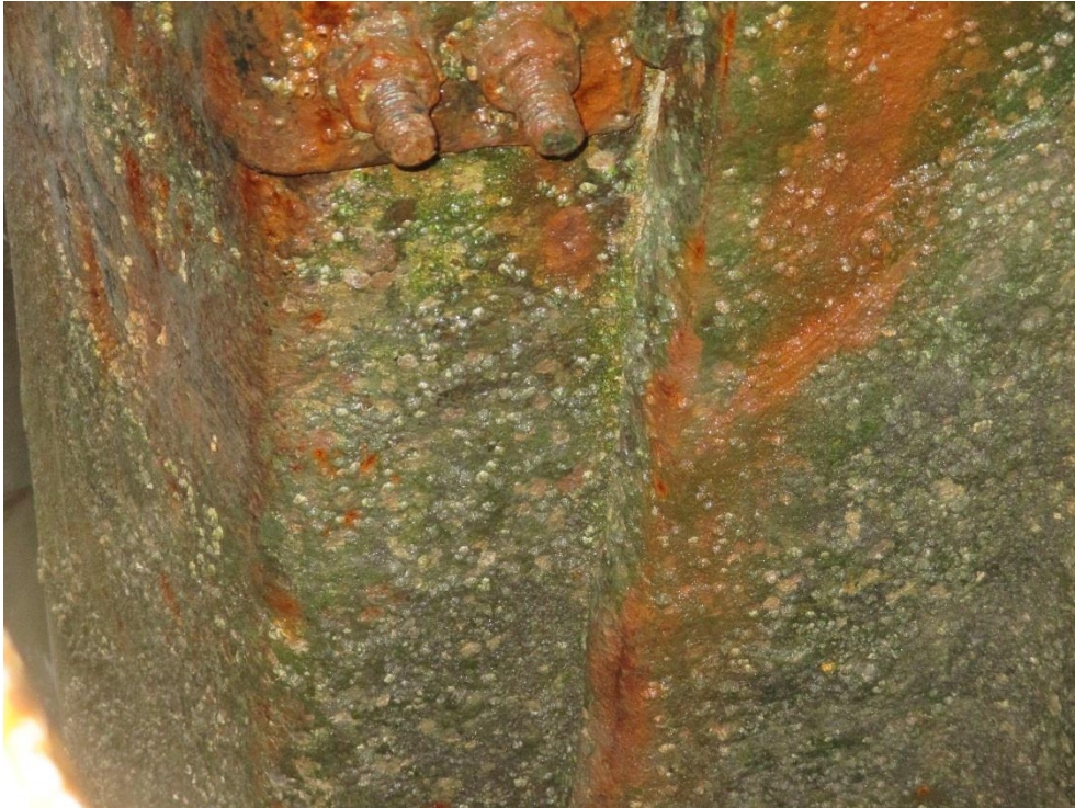
Fig B11 - Typical Condition within Intertidal Zone, beneath repair plates.
