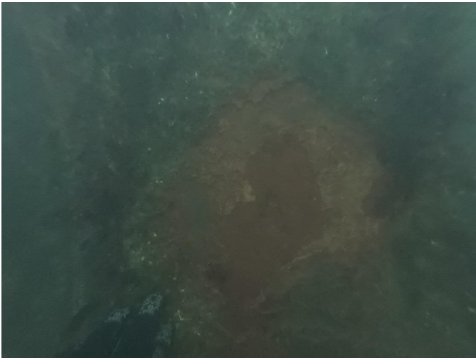
Fig B20 - Typical Active Corrosion at MLWS
