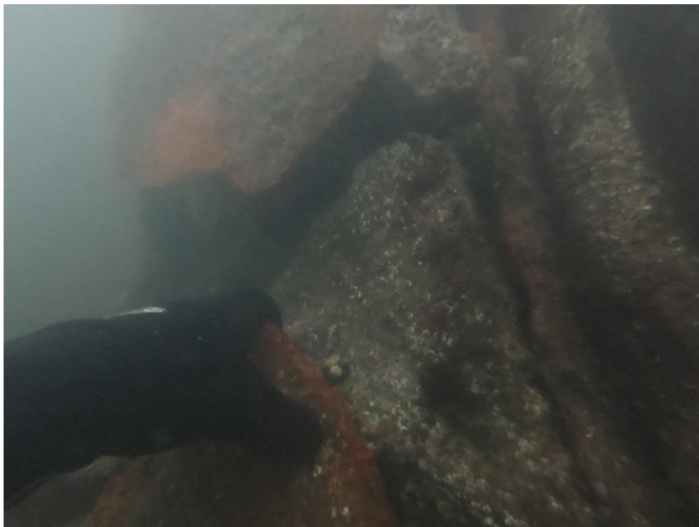
Fig B26 - Thin remaining steel / Loose fill stone within – Typical detail
