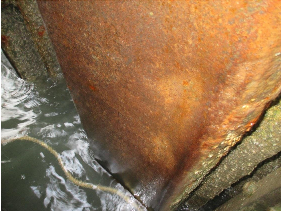
Fig B15 - Typical Steel Surface condition within intertidal zone along South Berth face
