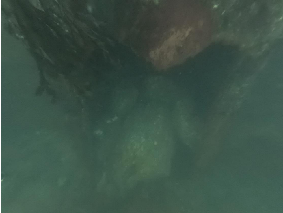
Fig B19 - Hole at bottom of Outpan No. 15 – Northeast Wing
