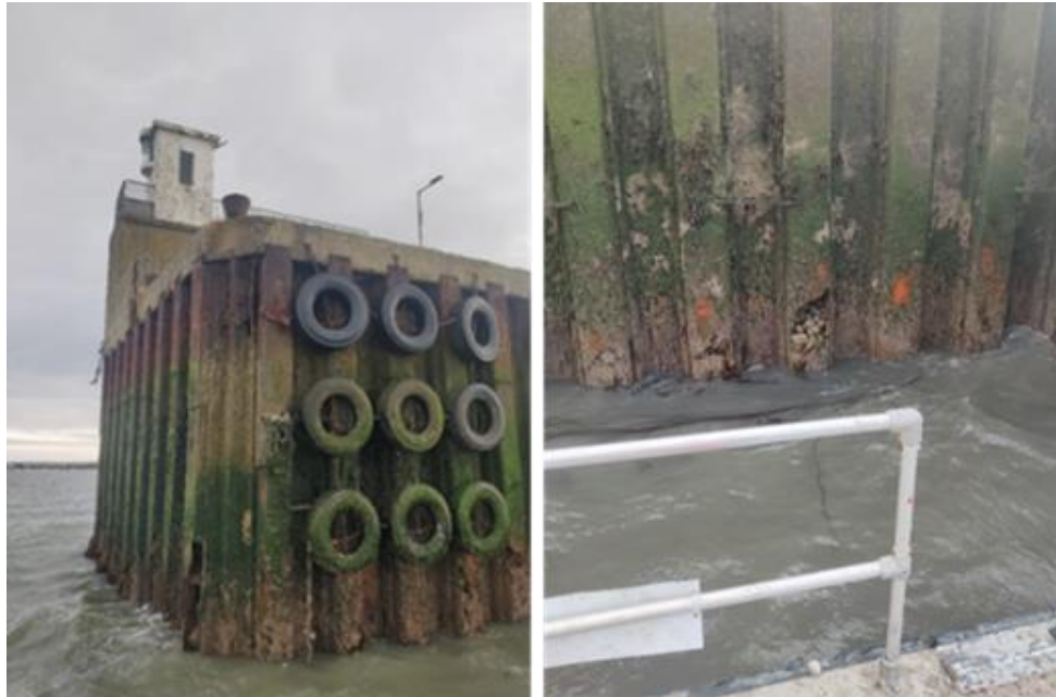
Figure 1-5: View of the Sheet pile pier and the extensive corrosion.
