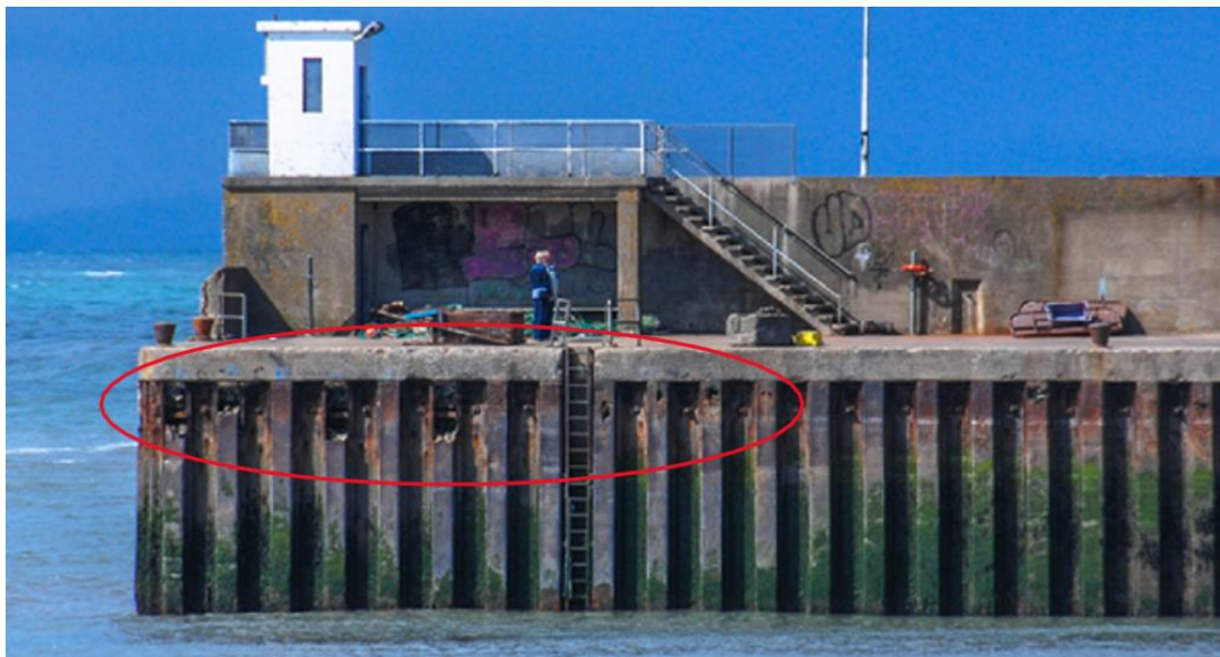
Figure 2-3: Photo of Sheet pile Corrosion Circa 2005 (source eOcenic [1])
