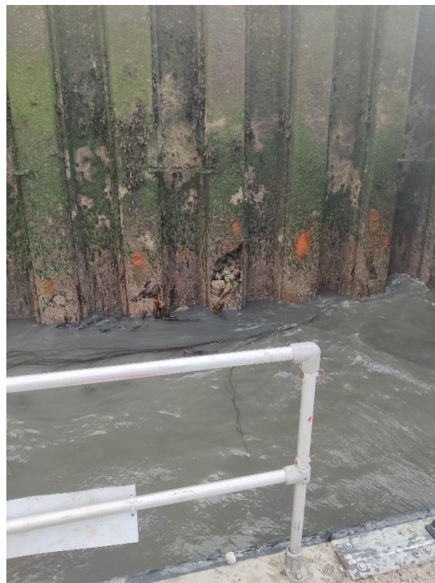
Figure A-2: Rock Infill Spilling from Existing Corrosion Holes.
