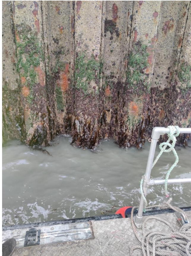
Figure A-9: Extensive Marine Flora Growth at the Lower Tidal Ranges of the Sheet-Pile Wall.
