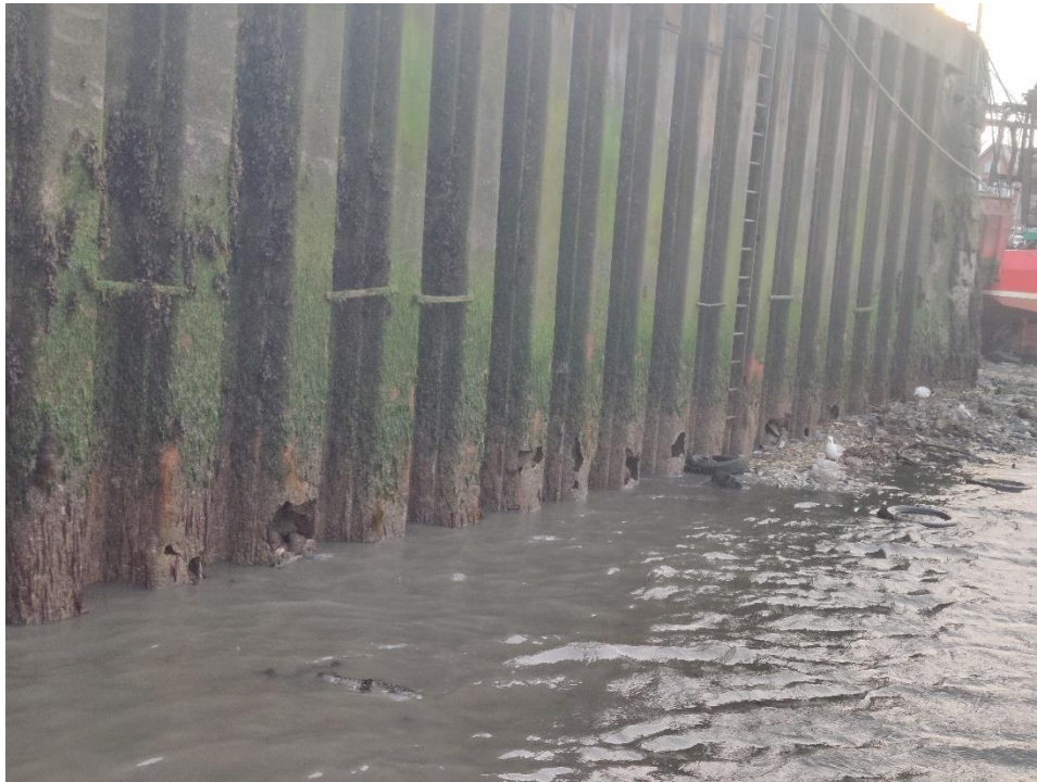
Figure A-1 Corrosion Holes Present at the Lower Tidal Water Levels of the Sheet-Pile Wall on the Leeside of the Pier.
