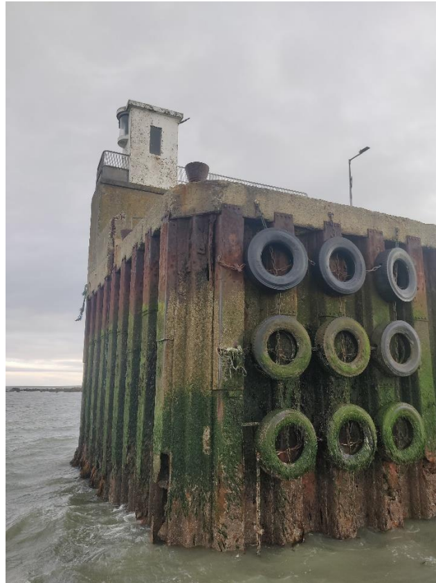
Figure A-3: Corrosion of Sheet-Piles at the end of Skerries Pier.
