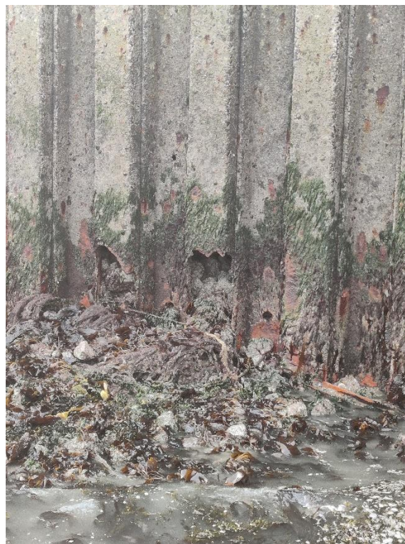
Figure A-10: Corrosion Holes in the Sheet Piles on The Seaward Side of the Pier
