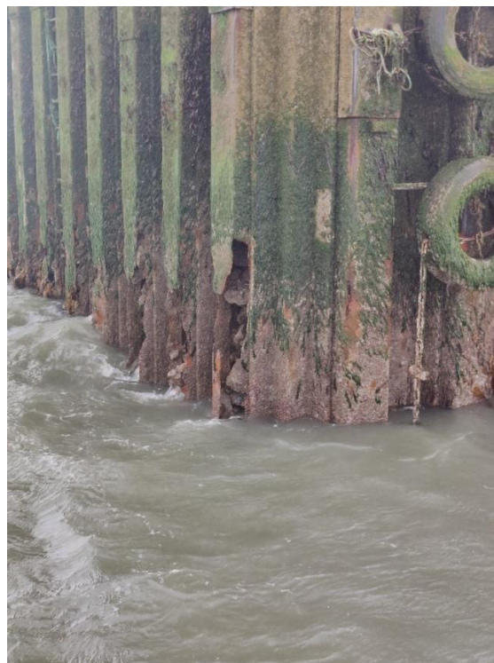
Figure A-4: Corrosion Holes & Rock Infill Spilling Present at the Lower Tidal Water Levels of the Sheet-Pile Wall on the at the End of Skerries Pier.
