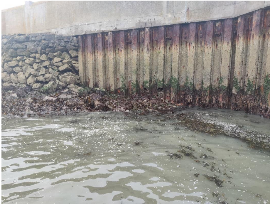
Figure A-11: Corrosion Holes in the Sheet Piles on The Seward Side of the Pier
