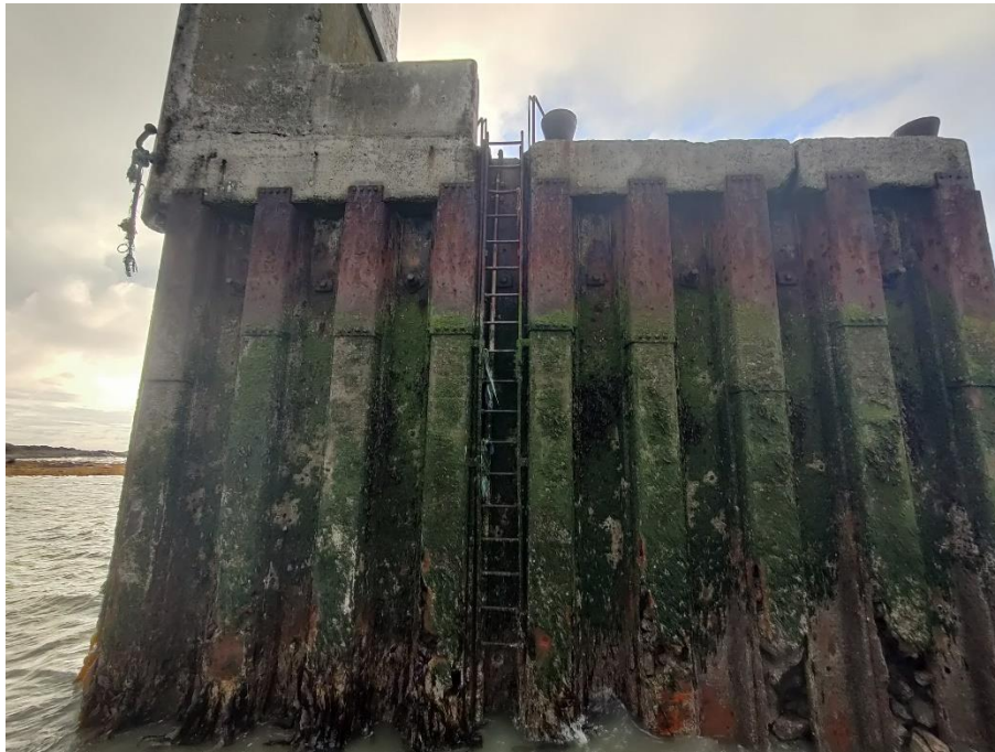
Figure A-5: Corrosion of Sheet-Piles at the End of Skerries Pier.
