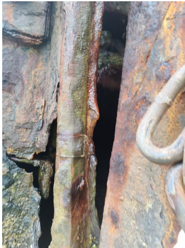
Figure A-6: Complete Corrosion at the Top Sheet-Pile Wall at the End of Skerries Pier.
