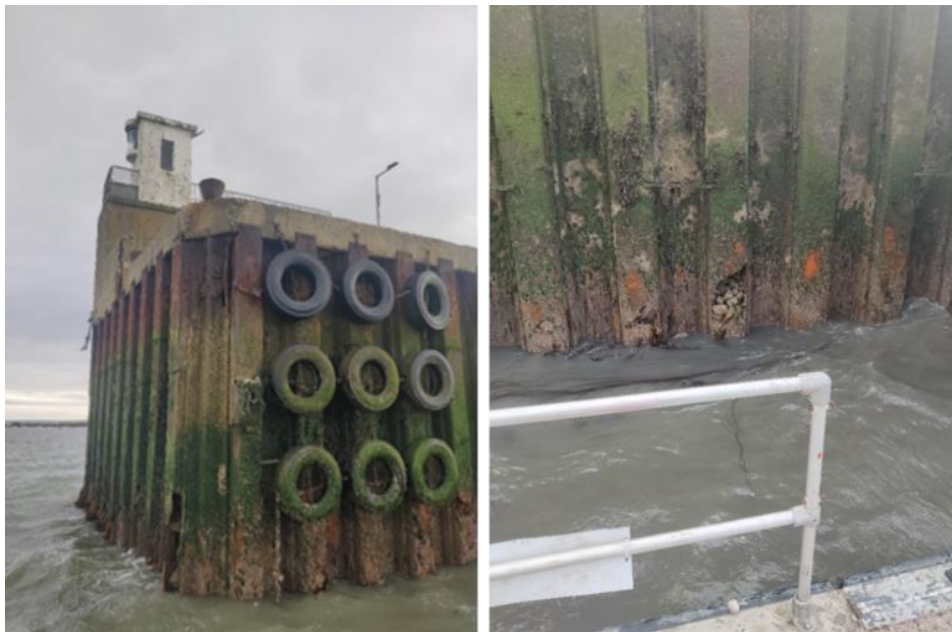
Figure 2-4: Photo of Sheet Pile Corrosion
