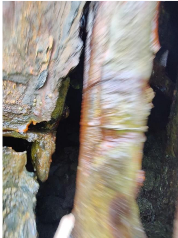
Figure A-7: Void Behind the Wall at the End of Skerries Pier.
