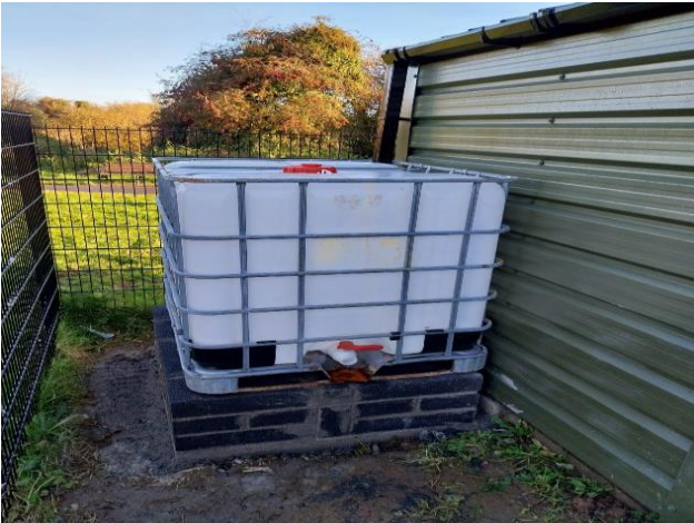
Newly installed Rainwater harvesting container at Broadmeadow Community Garden as part of 2023 programme of Works.
