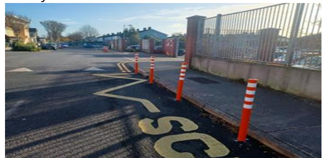
Below: New Plastic Bollards and Double Yellow Lines installed outside entrance to Scoil Neasain - Baldoyle
