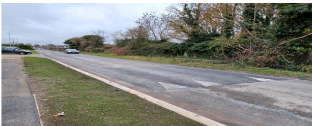
Five ramps Installed along Chapel Road -Kinsealy following activation of the Street Lights on the 20/11/23
