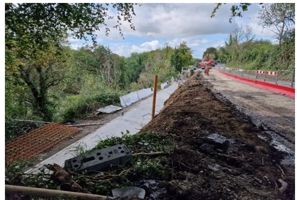
The next stage of reconstruction of the Brackenstown Rd is now underway. The image shows the foundations cast for the support of the embankment.
