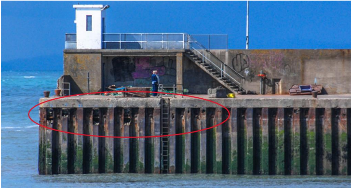
Figure 1-7: Photo of Sheet pile Corrosion
