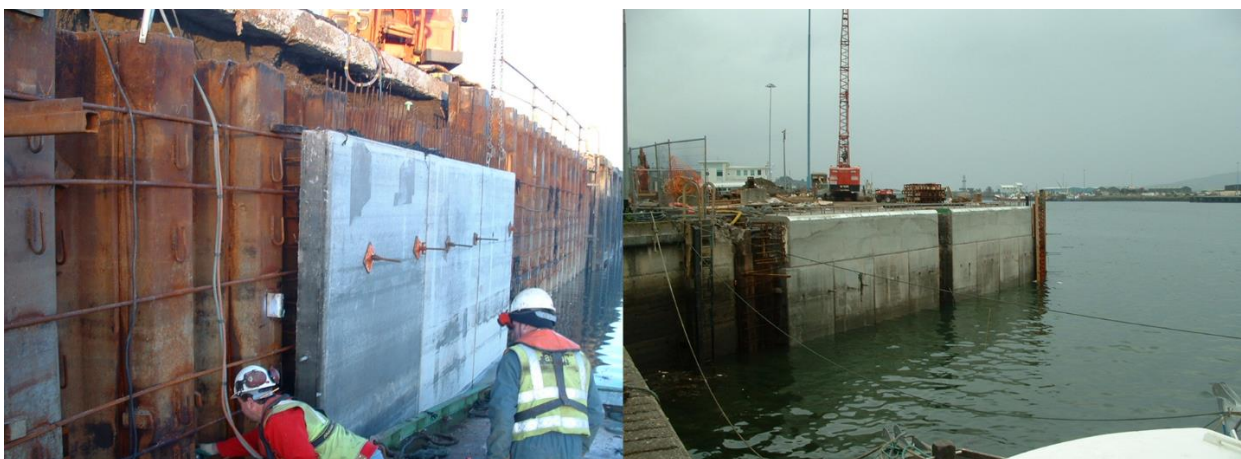
Figure 8-3: Concrete Panel being Installed (Left) and Finished panelling and Capping Beam (Right)
