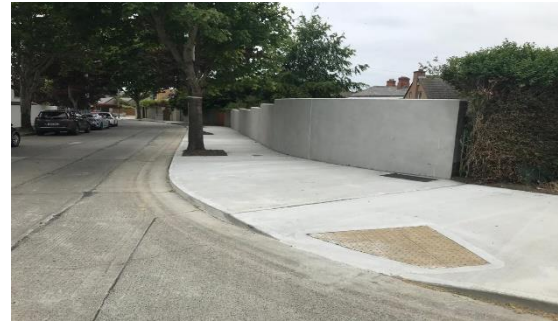
Footpaths replaced and drop kerb and tactiles installed at Glencarraig, Sutton by crews
