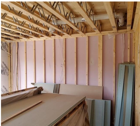
Checking web joists and timber frame in a housing development in Clonsilla.
