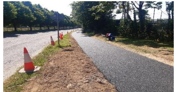
Before and after photos of new footpath inserted along back wall of Recycle Centre Porters Road at fire station Coolmine
