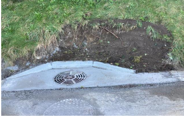
Recessed perforated manhole sump
