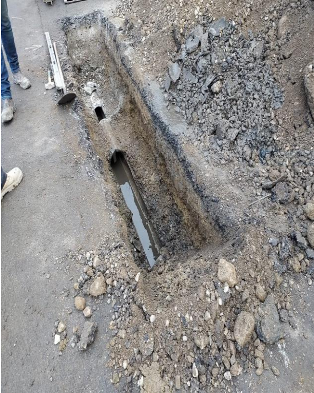
Before - collapsed concrete pipe
