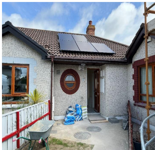
Successful solar panel installation
