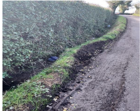
Road subsidence – Palmerstown
