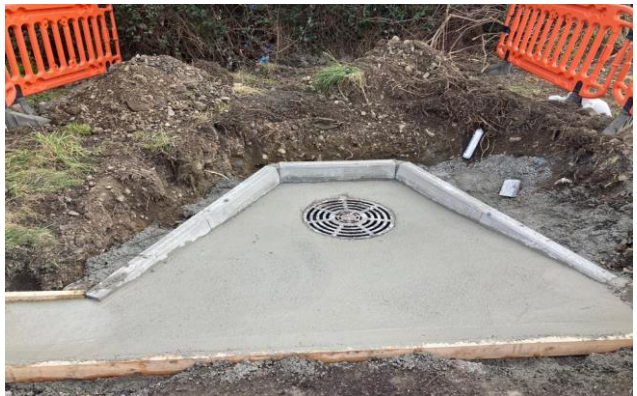
Recessed perforated manhole sump
