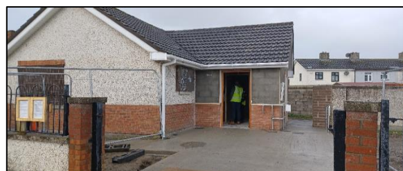
Extension works progressing on Council property in accordance with the Disabled Persons Grants Scheme
