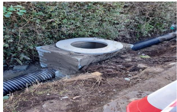
Piping of open channel section of drain
