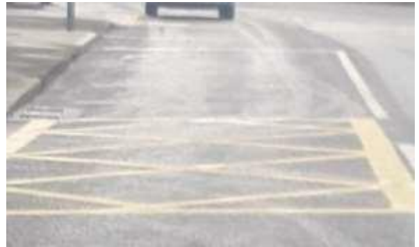
A newly installed yellow box on Shelerin Road outside Global Service Centre
