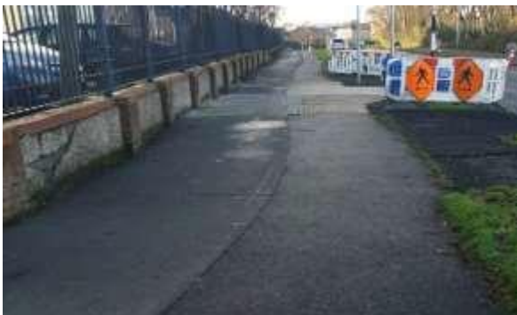
The upgrade of the existing junction at Hayworth Drive adjacent to Castaheany/St. Benedicts school has been completed. The contractor has also upgraded the existing zebra crossing to enhance
