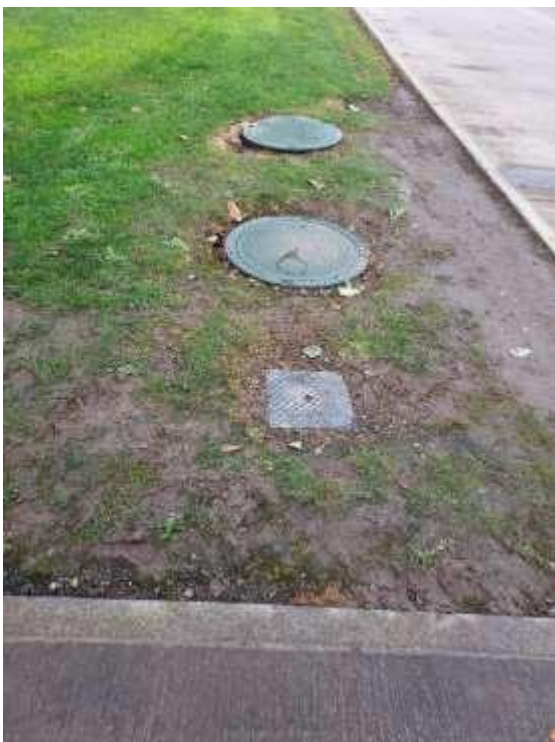
Commencement of drainage works for foul sewer repair at Balgriffin Burial Grounds
