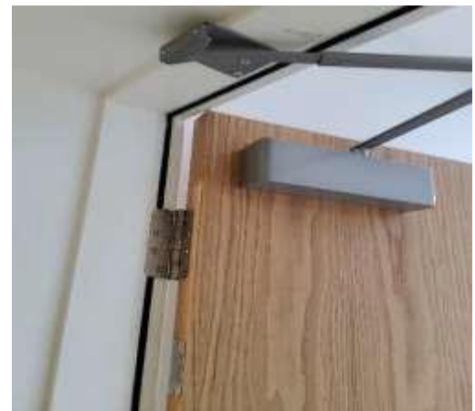
30-minute fire door into apartment with intumescent strip, cold smoke seals, self-closer and fire door stamp
