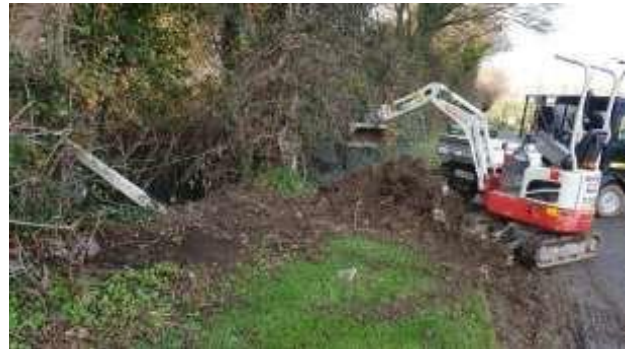
Winter hedging clearance being carried out above with a mini digger to assist at Balgriffin Cemetery
