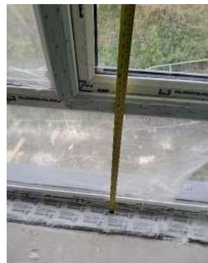
Checking height of window opening on a house in Dublin 15 for compliance with Part K of the Building Regulations
