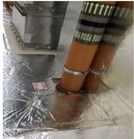
Service going through wall with fire collar and sign off sticker from fire subcontractor
