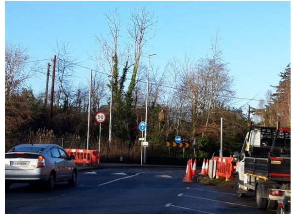
Works in progress for the new pedestrian crossing on Old Hansfield Road
