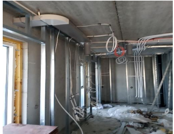
Inspecting fire sealing of services passing through walls on a site in Carpenterstown.
