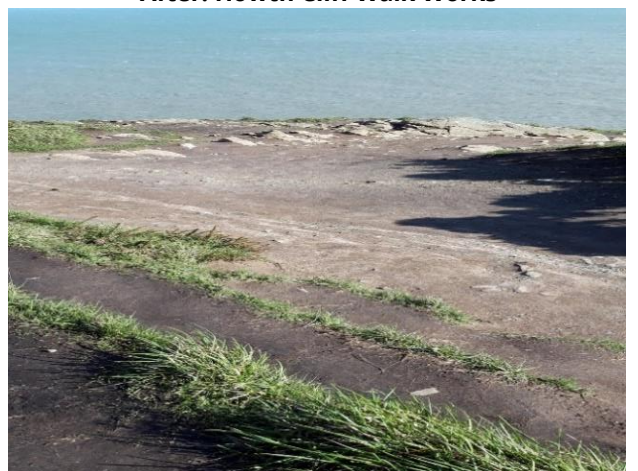
Rough ground at viewing area making it difficult to access this area.
