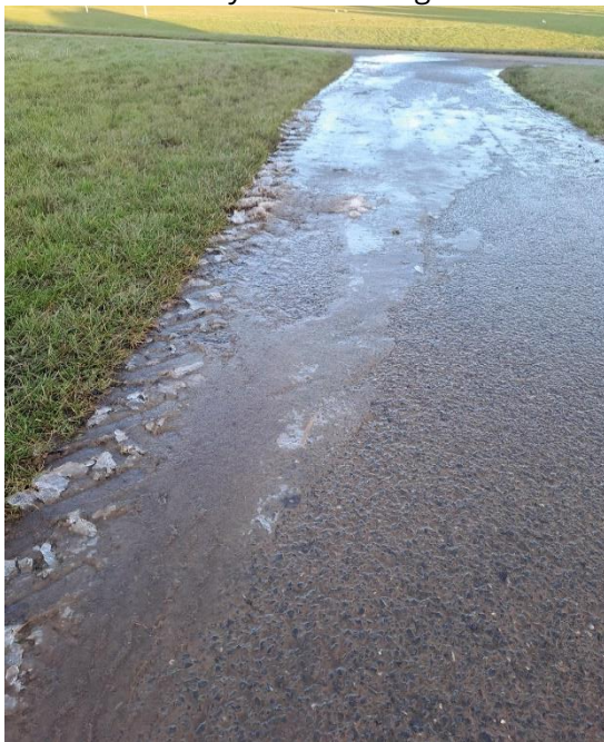
Example of flooding before Drainage works
