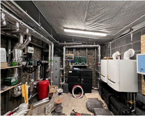
Inside of New Boiler House for Butterfly House
