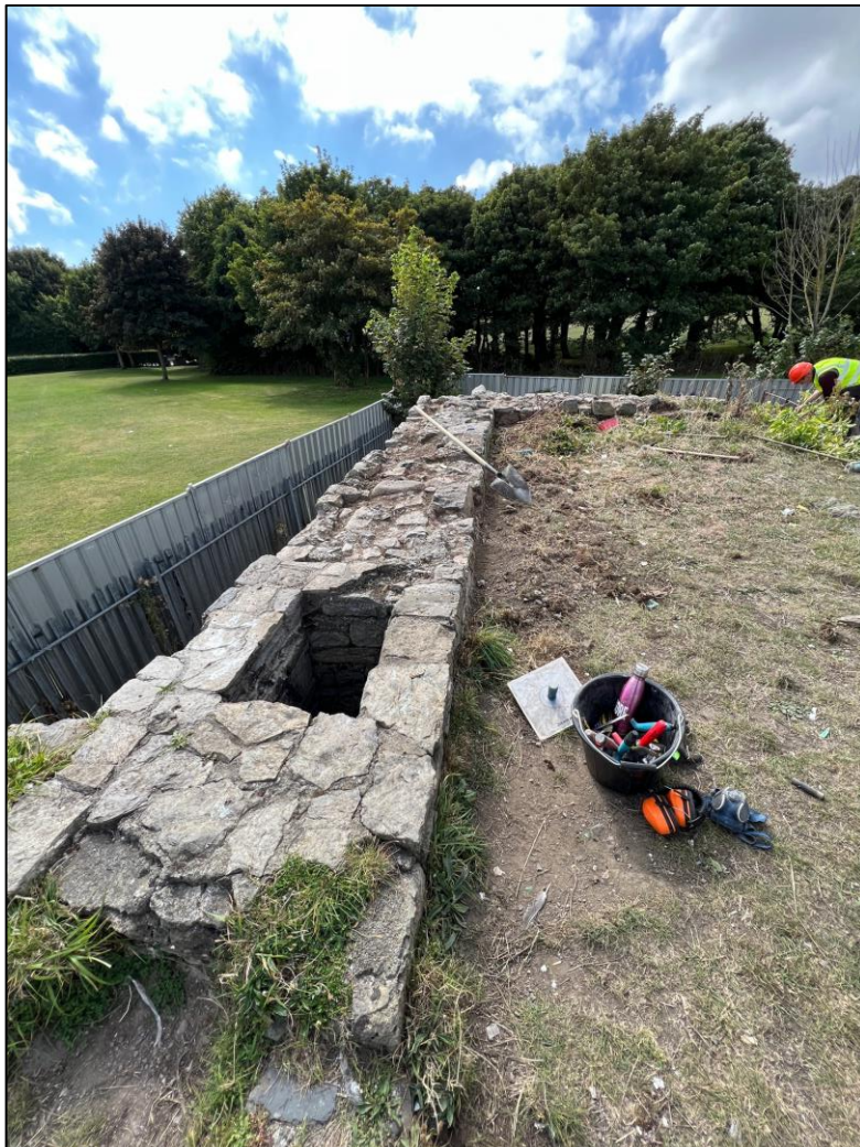
Plate 6 Vegetation removal from top of vault, facing west
