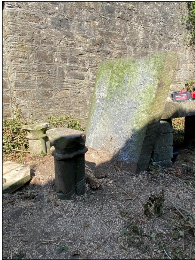
Plate 4 Northwestern column repair of table tomb interior of church
