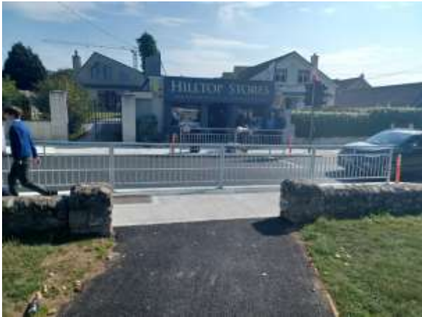
New pedestrian barriers and tactile paving to improve safety at exit from St Sylvester's Villas to R124
