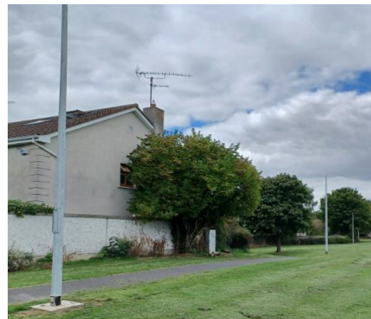
Phase two of Pine Grove, Swords trial motion activation lighting system under construction
