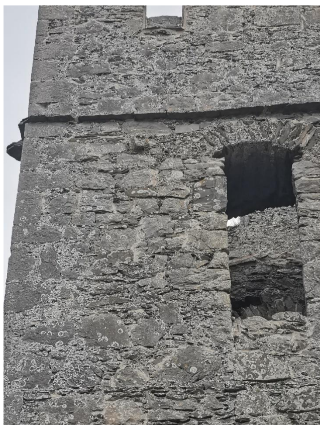
Plate 56: 12.2, face on south face of St. Catherine's bell tower
