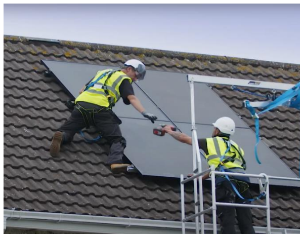
Solar panels being installed as part of the Social Housing retrofitting program.
