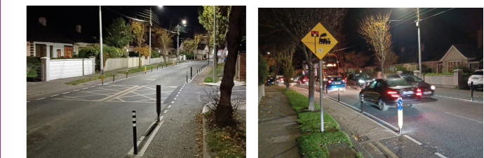
Baldoyle - Howth Protected Cycle Lane Scheme: Bollard installation on upgraded cycle lanes on Grange Road & Warrenhouse Road.
