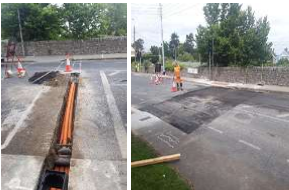
Upgraded pedestrian crossing installed at Howth Road/Offington Park Junction including reinstatement works.
