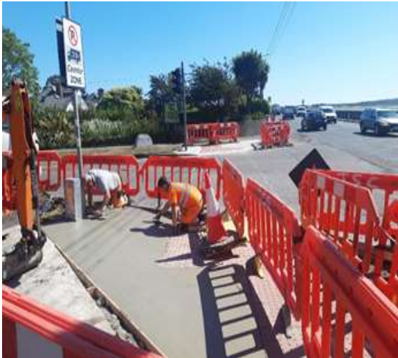
Ongoing works at Bayside Boulevard and the Dublin Road for new pedestrian crossings and updated signal control system (MOVA)
