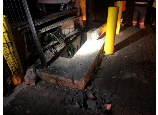
Uprooted protective bollards and upturned ESB sub-station
