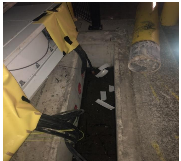
Exposed cables and fittings made safe by ESB crew
