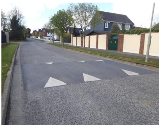
Remarking of all the Sharks Teeth on the ramps on Kettles Lane completed to assist with Traffic Calming
