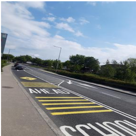
Road relining works completed on the Feltrim road by Scoil an Duinnígh
