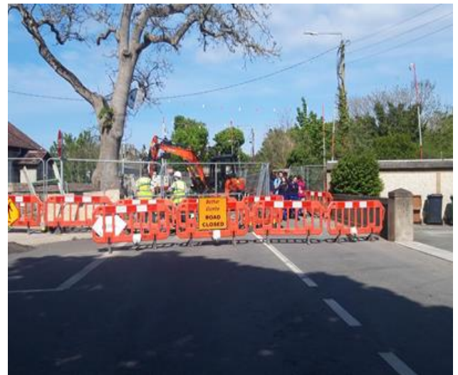
Works now completed by Irish Water Contractor on the Back Road which was closed by the Railway Bridge for a week earlier in May
