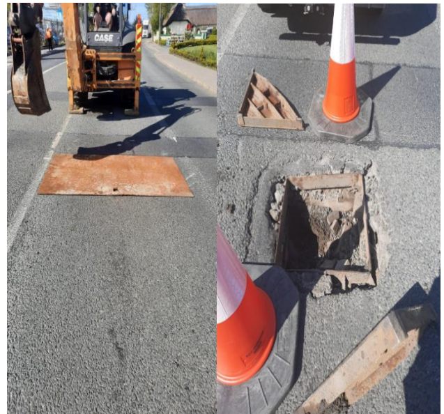
Failed asset covered by steel plate Failed chamber on the R132
