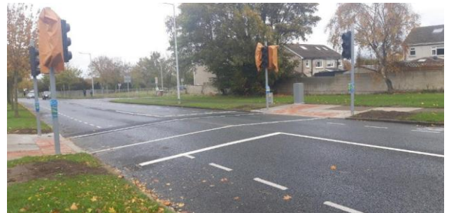
Newly installed Toucan Crossing - Civil works near completion. St. Cronan's Avenue, Swords
