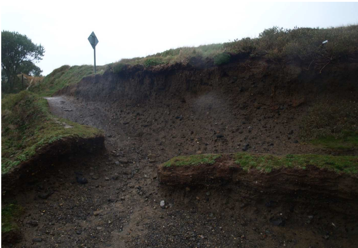
Figure 9: soil erosion due to excessive footfall on the cliff path
