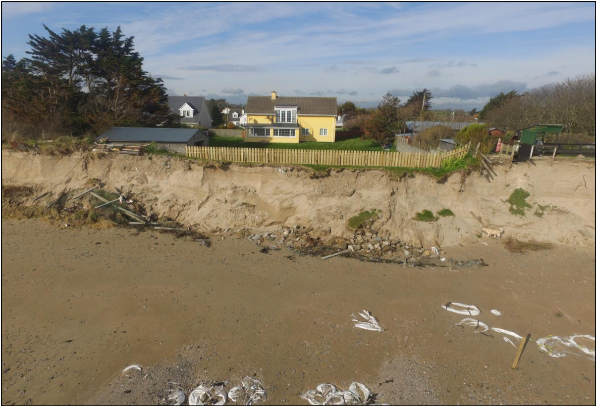
Figure 4.2: The severely eroded dune system and debris in front of residential property E.
