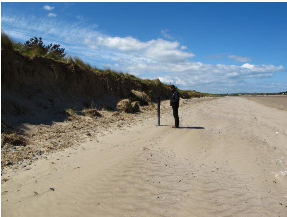
Figure 5.1.4: Eroding area, southern end of beach (looking north)
