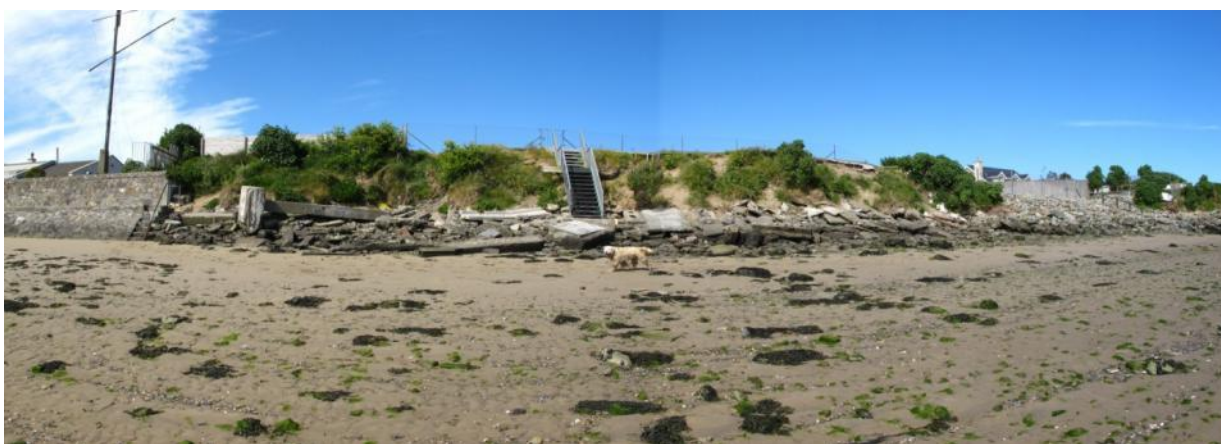
Figure 5.2.1: Rush boat club erosion and undermining
